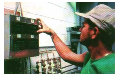
The MP90 microprocessor from Norcross allows the press operator to select and maintain virtually any viscosity control parameters desired. The unit activates alarms when viscosity levels reach high or low setpoints.
